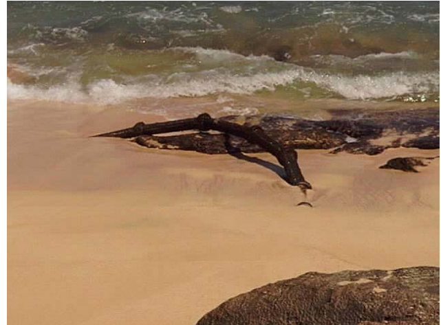
Figure 4 Split Pipe Failure at Southwest Bay, Ascension Island
